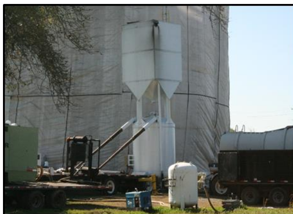
Blast Pot and Containment System
